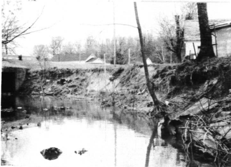
Figure 20. Bank erosion below Miller City Road box culvert
