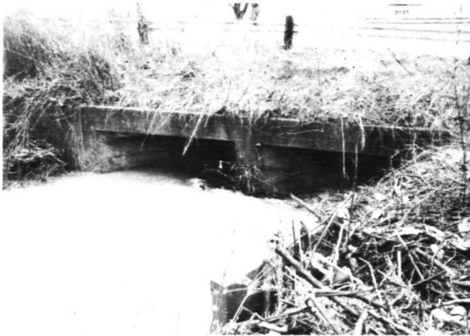
Figure 18. Flow entering Miller City Road culvert (Note proximity of water surface to the top of the culvert)
